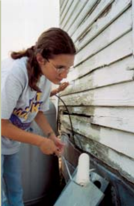
Jessie Pounds of Oak Ridge, Tenn., paints a farm worker housing unit.
