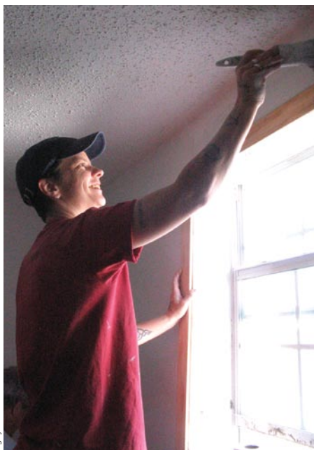
Eliza Galaher, intern and campus minister at the UU Church of Davis, Calif., paints inside a rebuilt home during UUSC’s JustWorks Gulf Coast camp in Biloxi, Miss.
